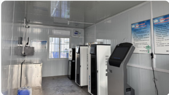
Wastewater online monitoring system equipment
